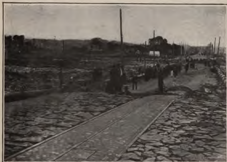
B. An area on Valencia Street, San Francisco, which was dropped and shifted laterally about ten feet. The damaged structures were consumed by fire.
